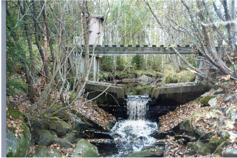
Figure 4. A weir structure for measuring the water level of a creek. Photo courtesy of SYKE.
